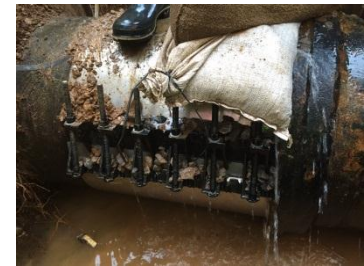
Leaking temporary repair clamp
